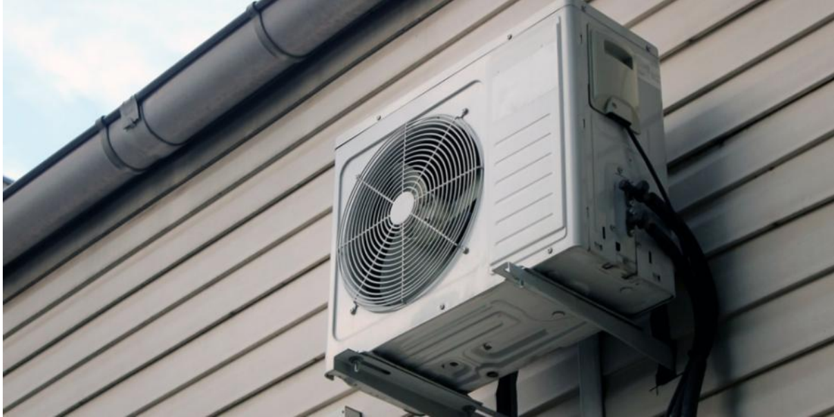
Figure 29: Small Domestic Heat Pump
